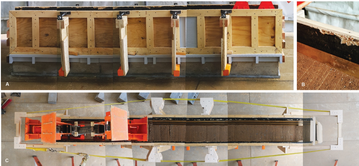
Figure 5: A novel machine for ramming earth requires formwork that is also somewhat atypical. Rotational Tamping formwork required external means of tensioning the sideboards of the formwork. At the lower level of the form this was achieved with mechanical adjusters that put inward pressure on the form (A). As the rammed earth wall grew and more layers of formwork were added, the top layers of the formwork were tensioned with heavy duty ratchet straps and wedges, as seen in the plan view (C). RT-01 also shredded the top edge of the formwork (B). Cutting it away at an angle allowed the square steel tramping plates to ease into the form rather than collide with the top edge as they entered the form cavity. Source: (Author 2023)
