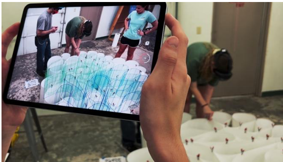
Figure 6: 1:1 prototype assembly process. Supervisors on the left are comparing the built form to the AR model and inspecting it for inconsistencies. Source: (Author 2024)
