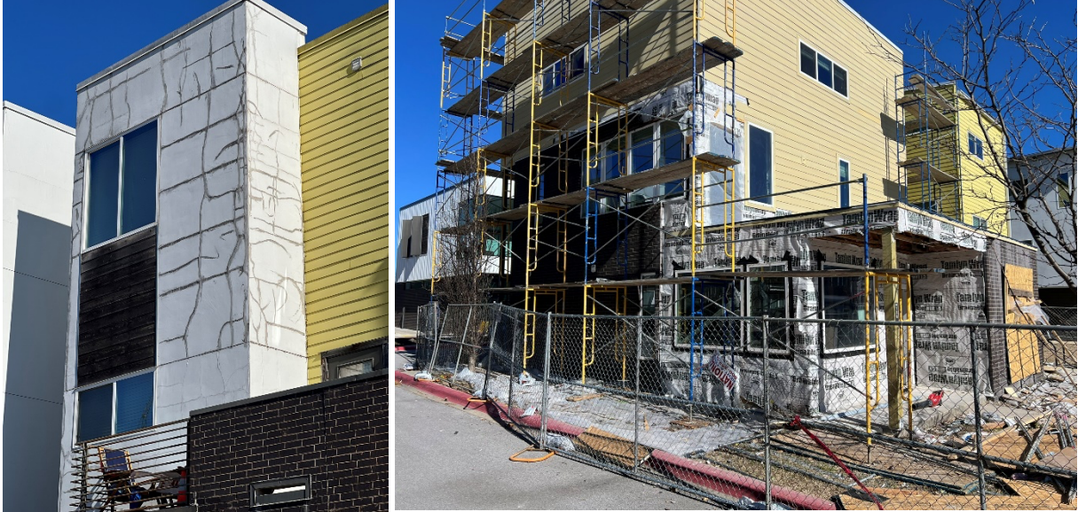
Figure 2: (Left) Envelope failures of typical new, market-rate housing construction in Fayetteville, Arkansas. Even when these failures permit continued occupancy of the structure, they degrade its value potential and portend more significant failures in the future. (Right) A typical, poorly constructed housing structure undergoing invasive repairs. The rapidity of construction, coupled with low-grade materials, catalyses building failures and triggers the need for repairs. This incurs extra expense, pauses revenue generation for the development’s owners, and takes an otherwise beneficial housing unit off the market. Source: (Author 2023)
