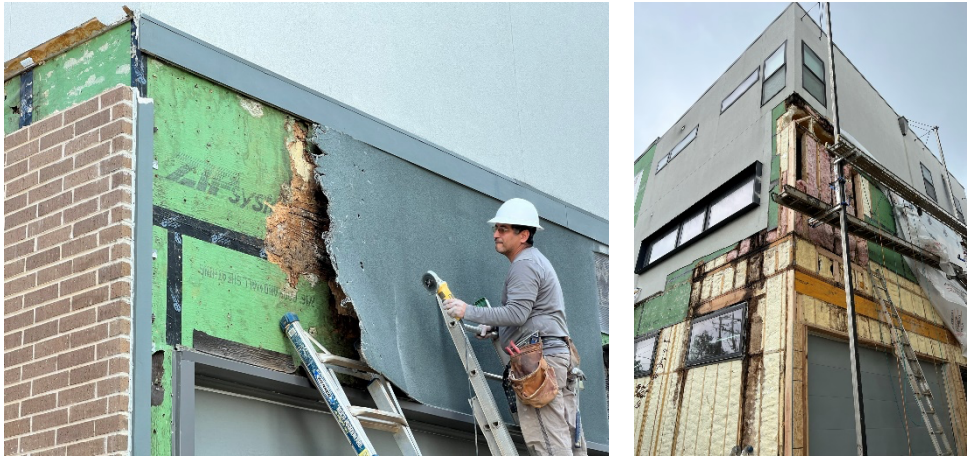
Figure 4: Stucco (i.e., portland cement plaster) comprised the plurality of facade materials. Its installation did not adhere to requirements established by building code and standards, dooming the defenseless wood structure behind. In the left image, damaged sheathing is exposed beneath the stucco. Where the yellow polyurethane insulation is visible, the sheathing has completely disintegrated. Source: (Author 2023)
