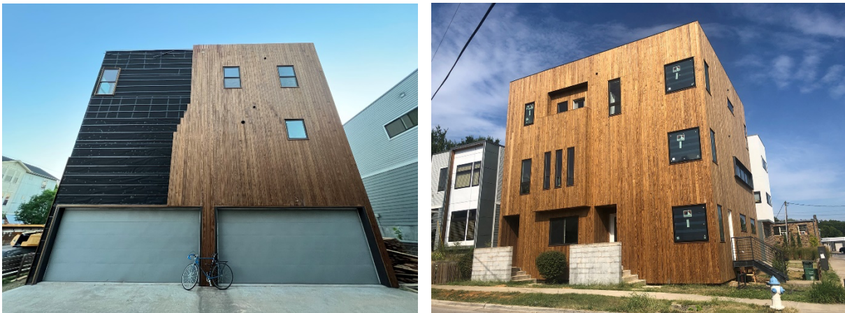
Figure 5: On the left, the non-adhesive, weather-resistive barrier and furring await coverage by the wood rainscreen. On the right, a corner perspective image of the completed building. Source: (Author 2023)
