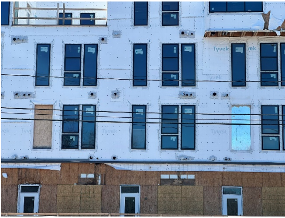
Figure 1: Incomplete multi-family construction on indeterminate hiatus in Northwest Arkansas. While they have latent potential for completion, the low-quality materials deployed cannot withstand long-term exposure. Source: (Author 2023)
