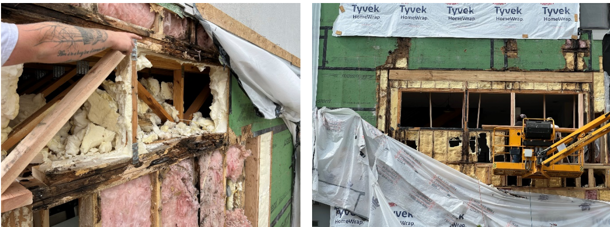
Figure 3: Water infiltration through the cladding and windows likely occurred for the life of the building. The polyurethane insulation is largely removed in this image to expose rotting structure, but its presence would have trapped the water, encasing susceptible wood members. Blackened structural members were completely friable; the material in this image was easily crumbled by hand. Sheathing and metal lath had completely disintegrated prior to demolition of the exterior cladding, making plain both the magnitude of the issue and the dangers it presented to human health and safety. Source: (Author 2023)
