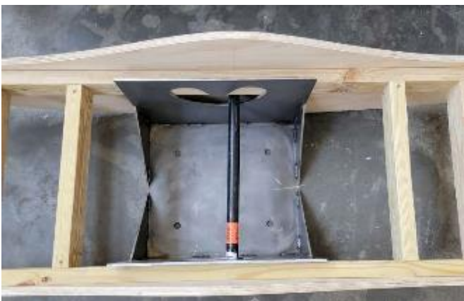
Figure 9: View of rocker anchor box with pin and slot to allow for movement. Source: (Dickey 2023)
