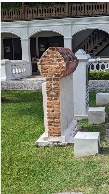
Figure 3: Masonry wall built from clay brick with white and red plaster on the exterior faces. Source: (Rutkowski 2023)
